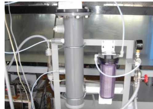
Water treatment unit (2 ton/day)
