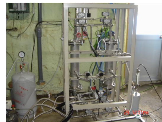
VPSA-CH 4 recovery and purification unit
