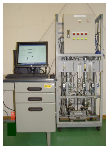
PSA-VOC recovery unit
