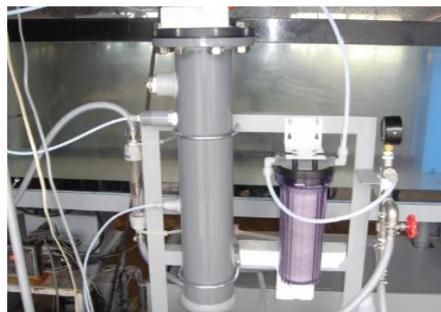
Water treatment unit (2ton/day) Sea water purification for cultivation
